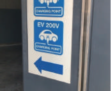
EV charging station
