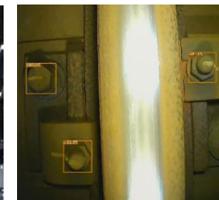
Use AI image analysis to check for loose bolts
