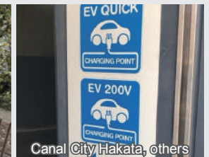
Canal City Hakata, others EV charging station
