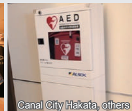
Canal City Hakata, others AED installation
